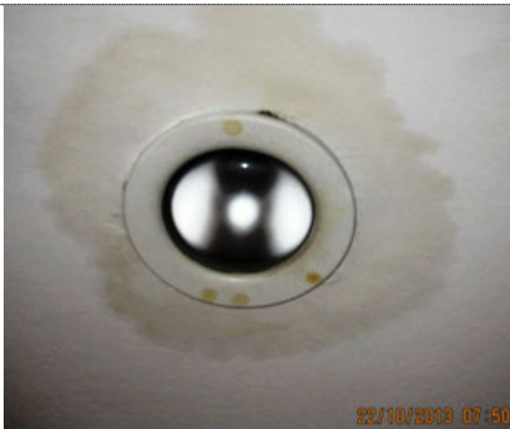
Photo of bathroom ceiling taken the following morning i.e. on 22 Oct 13
