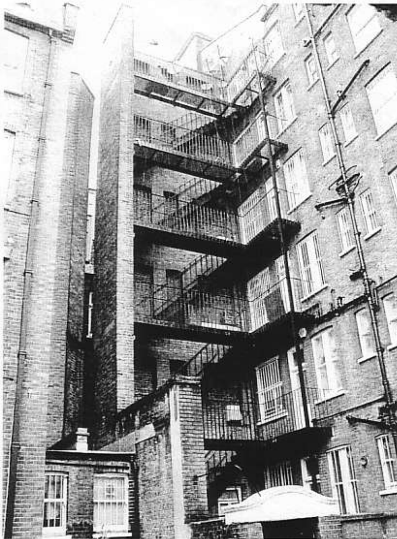
Top: view to Party Wall from Rysbrack St with infilled window openings
